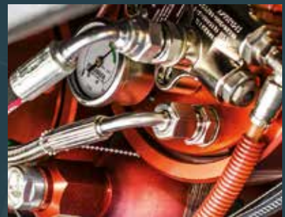
Extinguishing system and diesel particulate filter in accordance with tunnel construction requirements.
